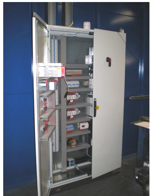
The control system
